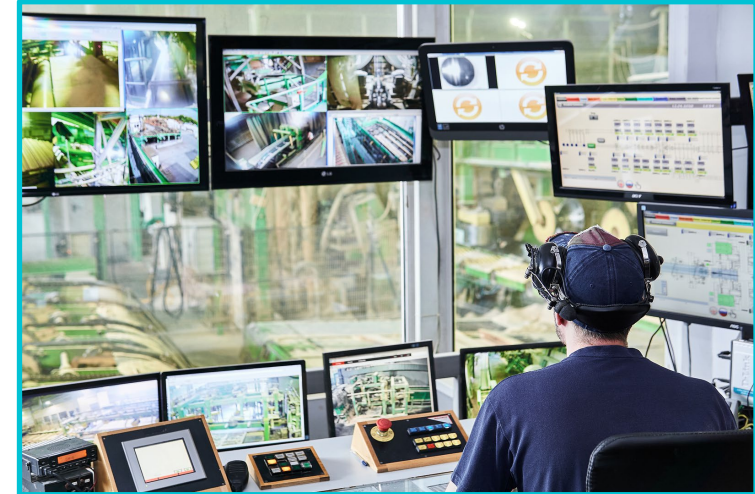
Controlling multiple components from a remote location
